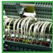
Electrical cabinets and substations
